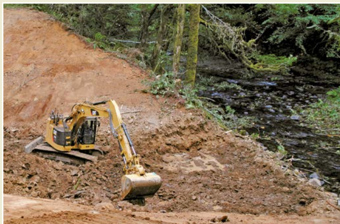
Above: Removing the railroad berm along the mainstream of the Upper Luckiamute River in the summer of 2013.
